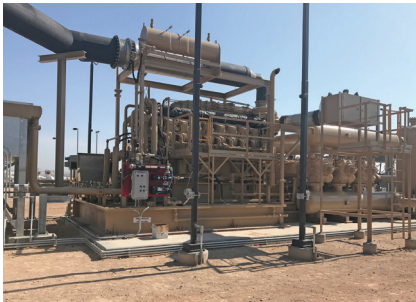
Gas compressor station
